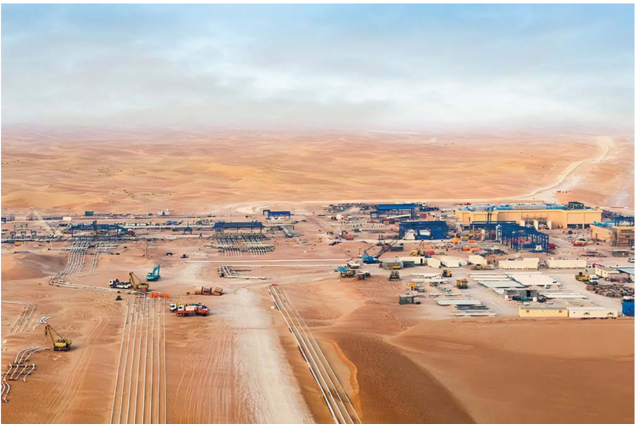
Haliba Field Development project of Al Dhafra Petroleum Operations Company Ltd UAE
