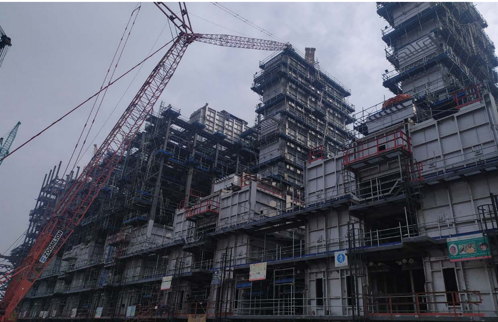
Cracker Furnace Package for HMEL Bathinda Refinery.
