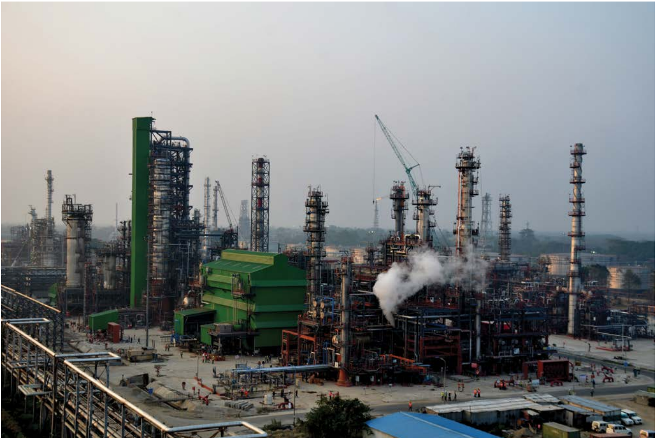
INDMAX FCC Unit including LPG Treatment Facility for IOCL at Bongaigaon, India
