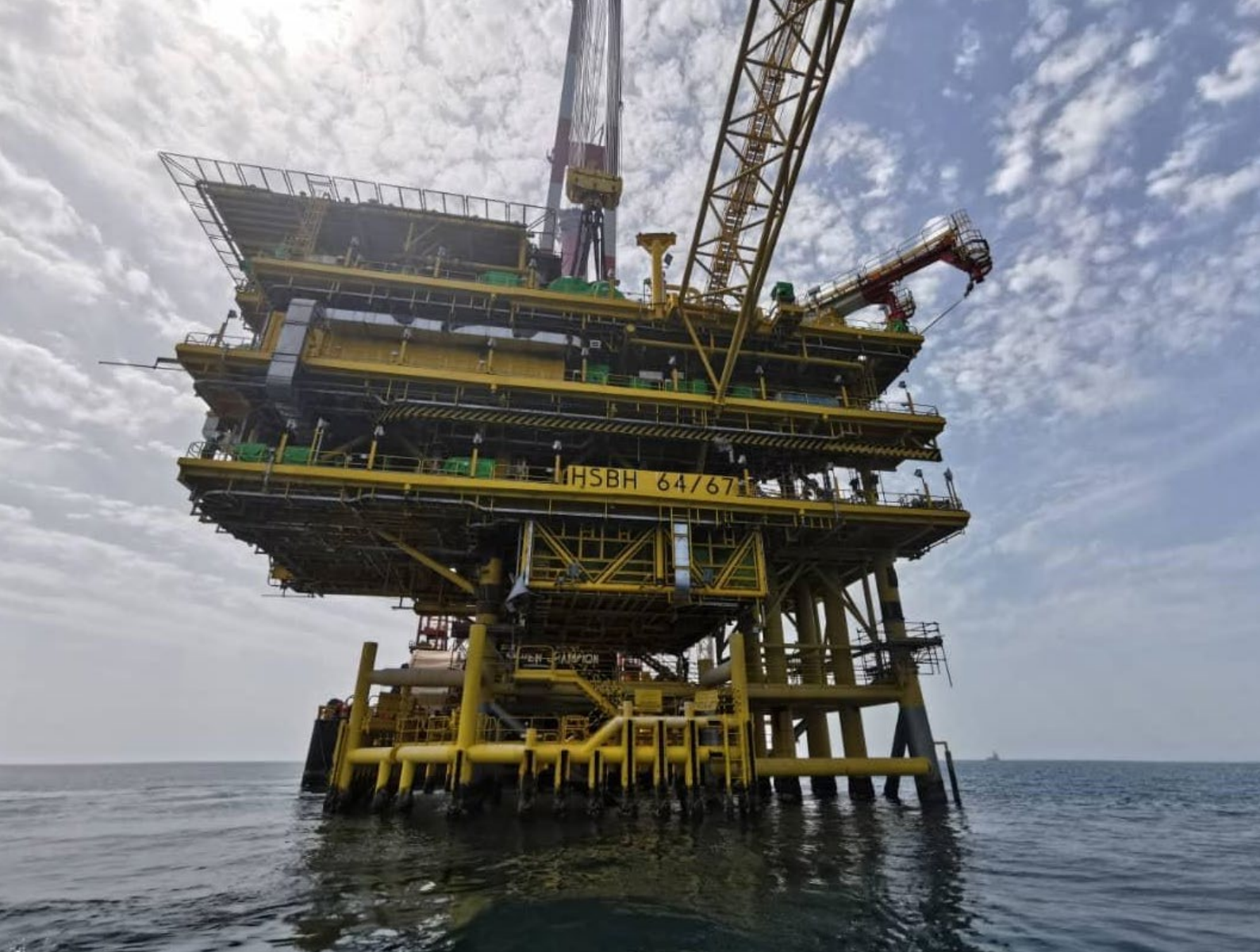
Gas PDMs installed in Hasbah and Arabia Offshore for Saudi Aramco.
