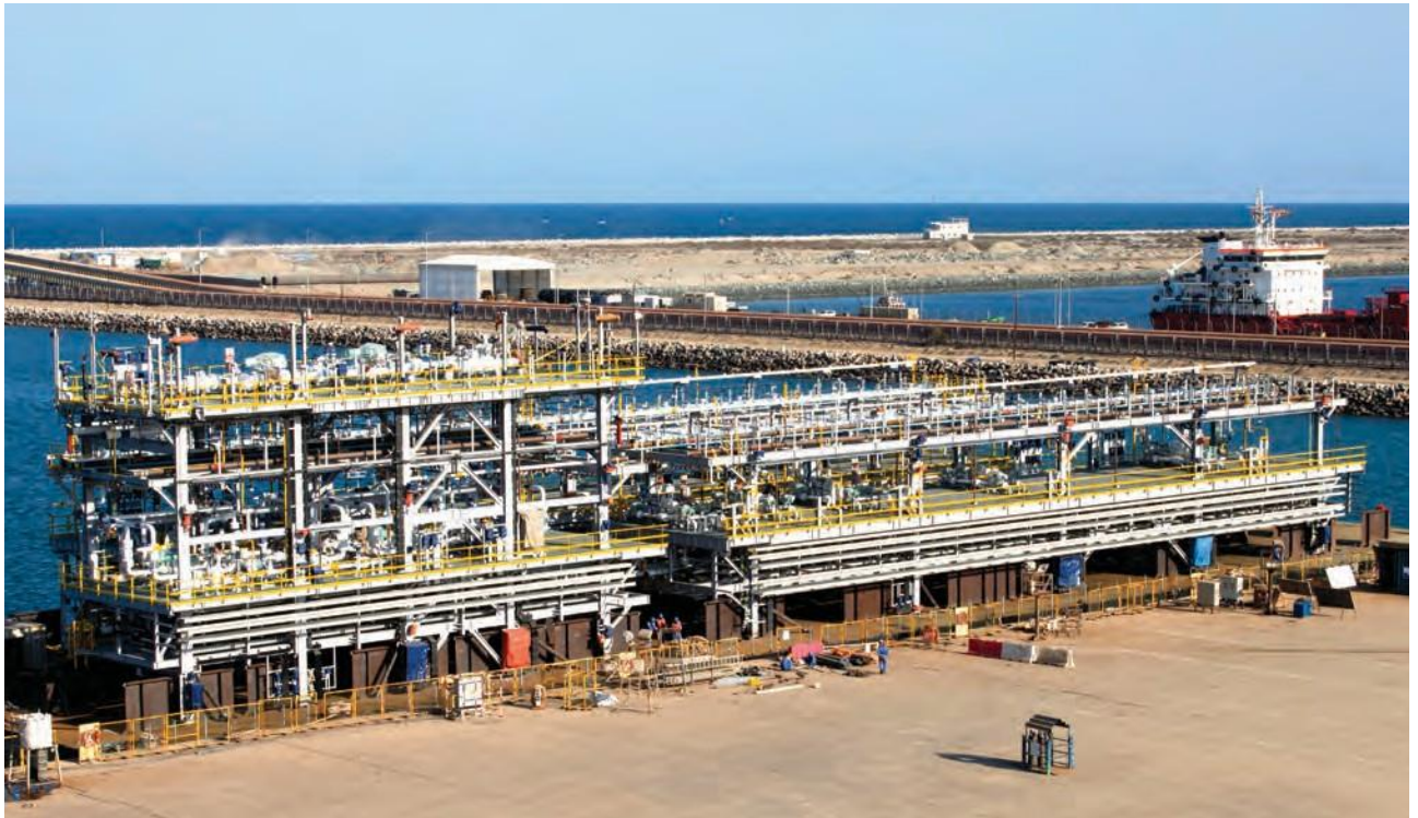
PAM and PAR modules for ExxonMobil / ZADCO's Upper Zakum Field development programme, ready for despatch at Sohar Yard in Oman. The scope includes engineering, fabrication and load-out of 33 modules weighing approx. 14,000 MT.
