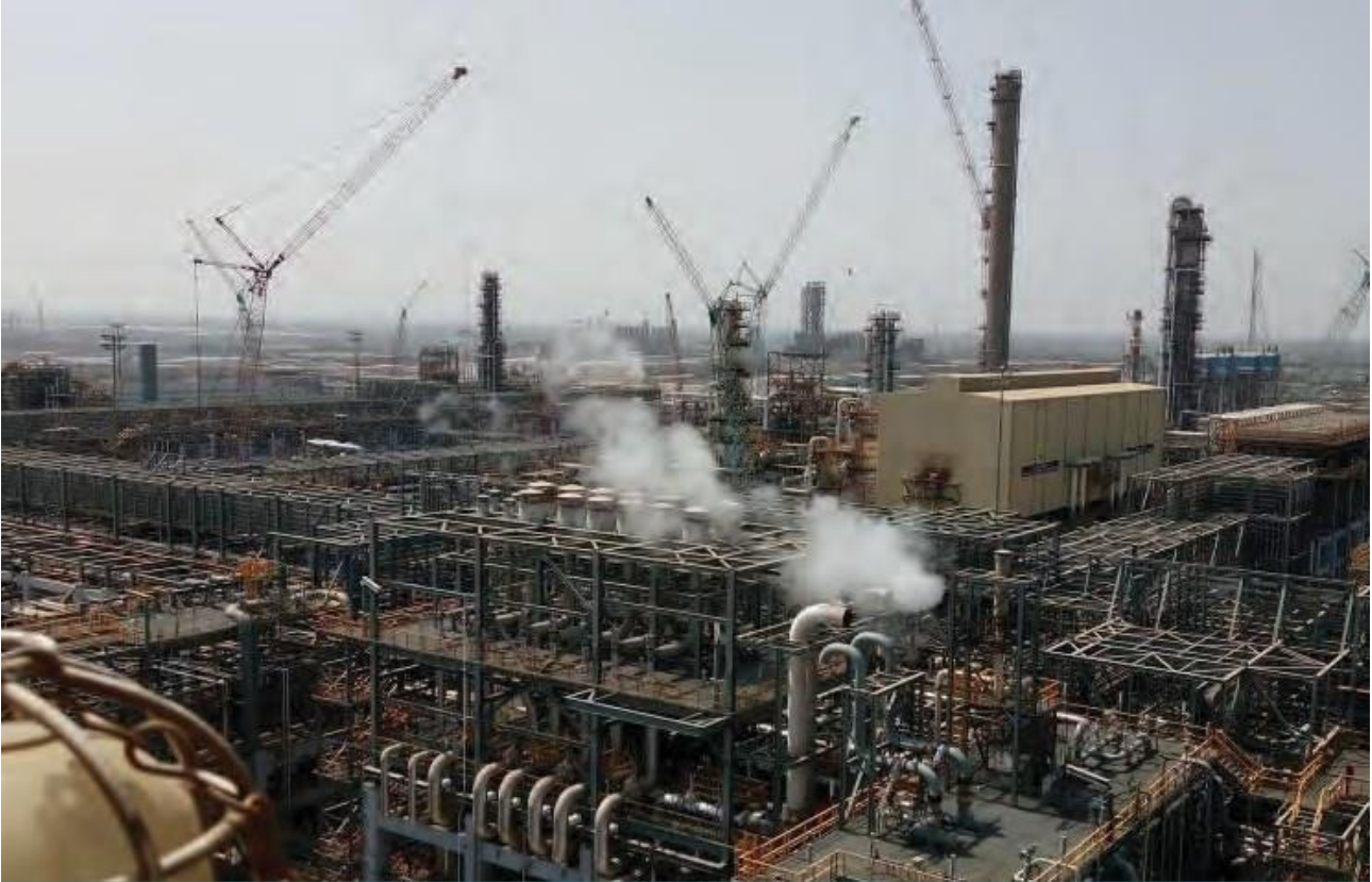
ROGC Plant at RIL Jamnagar Phase-III
