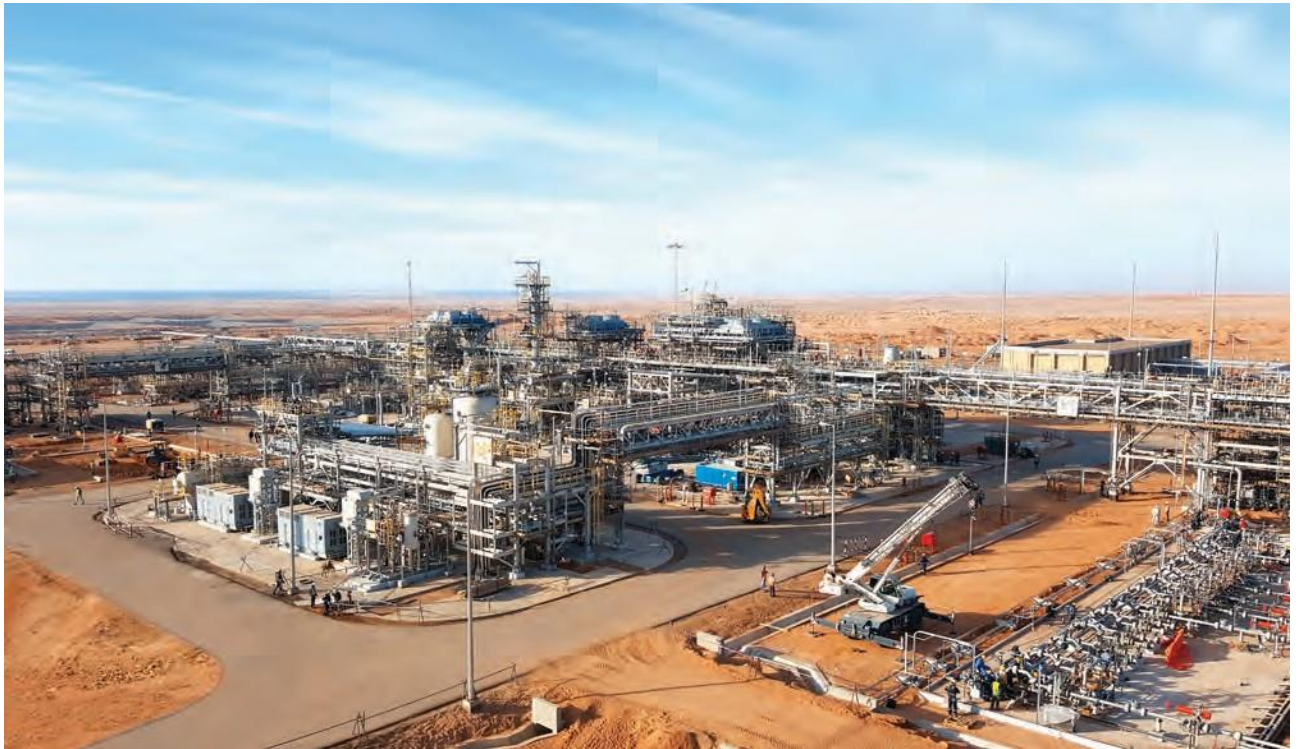
Gas processing facilities for Saudi Aramco near Tabuk in Saudi Arabia, with a capacity to treat 75 MMSCFD of gas and 4500 BPD of condensate, and the laying of over 90 km of gas and condensate product pipelines.
