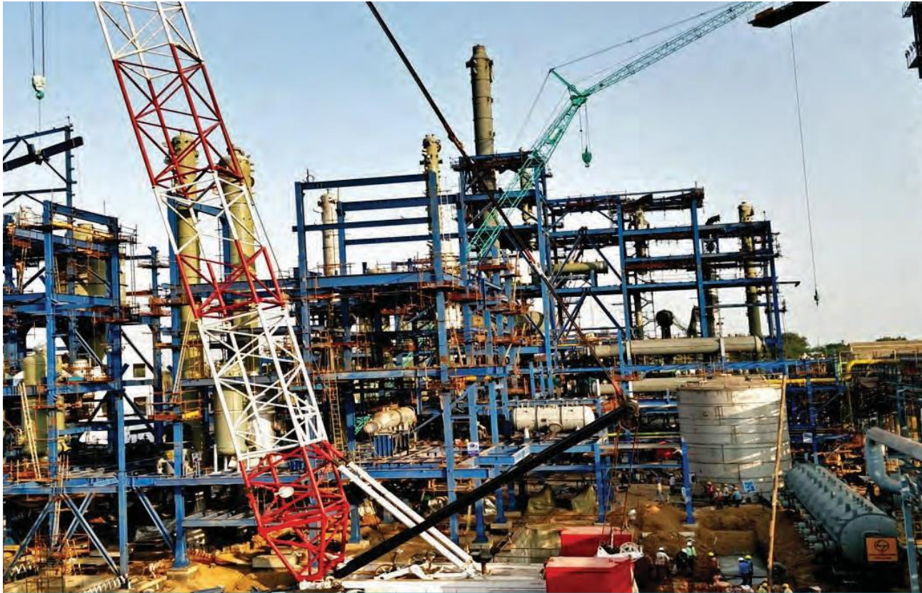
40000 MTPA MELAMINE PLANT for GSFC in Baroda, India
