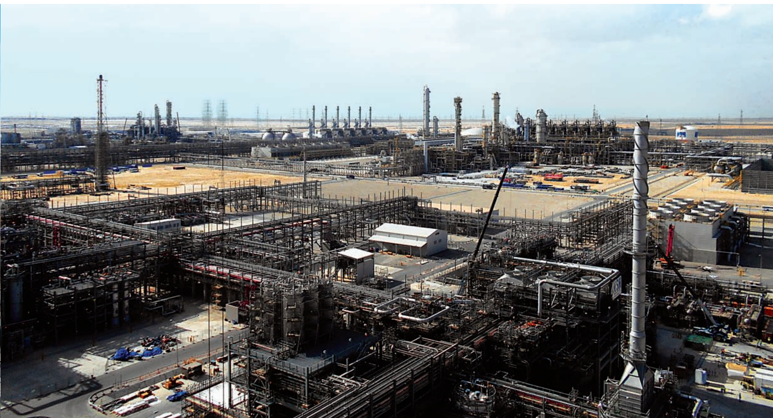
Construction of Polyethylene Trains for SADARA Chemical Company (JV of Saudi Aramco and Dow Chemicals) at Al Jubail, Saudi Arabia
