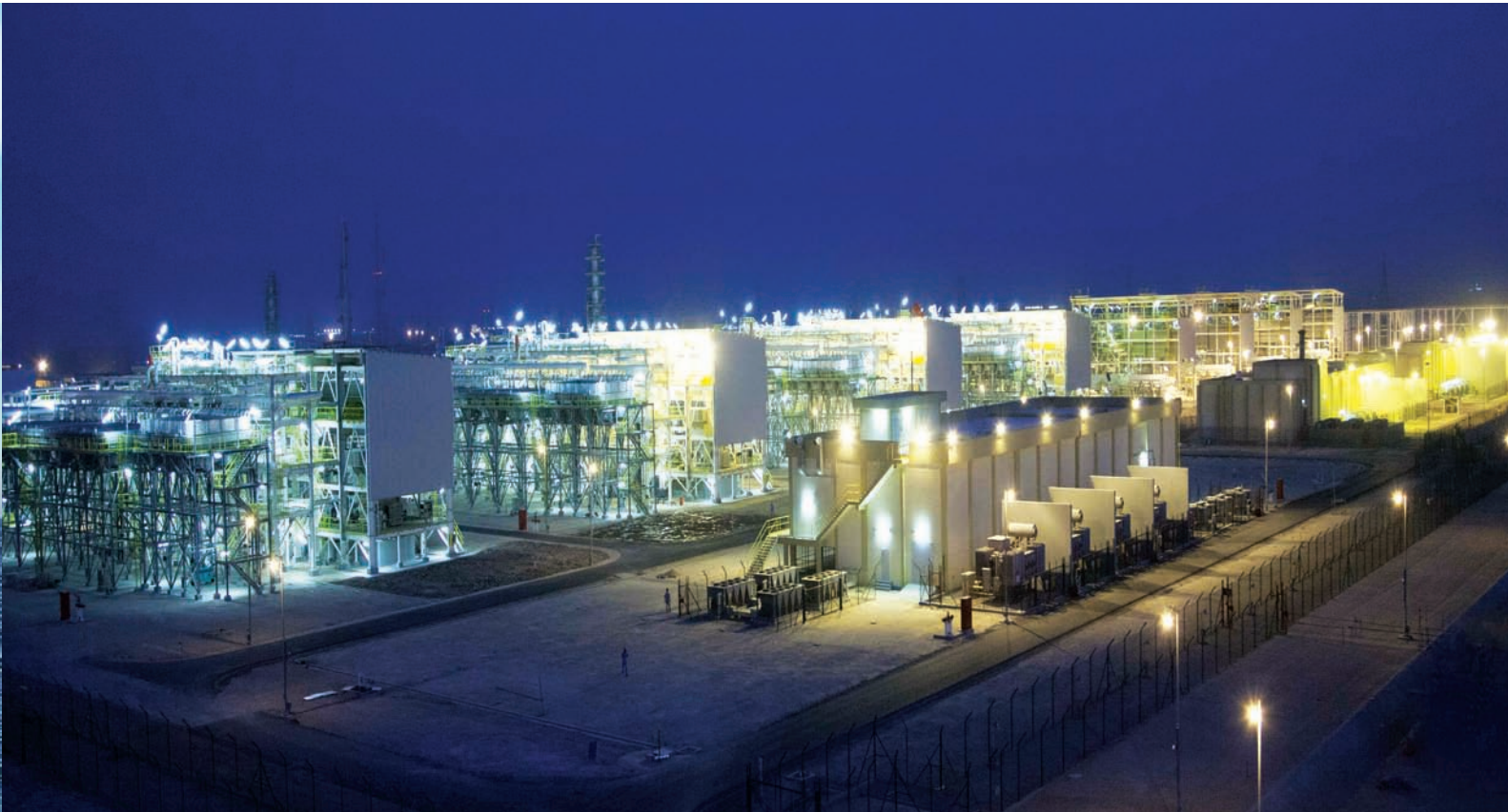
Saih Rawl Depletion Compression Phase 2 (SRDC2) for Petroleum Development Oman (PDO). The Company has also built PDO's gas processing facilities at Lekhwair and Yibal, and is executing its SNDC2 and KDC2 gas compression projects
