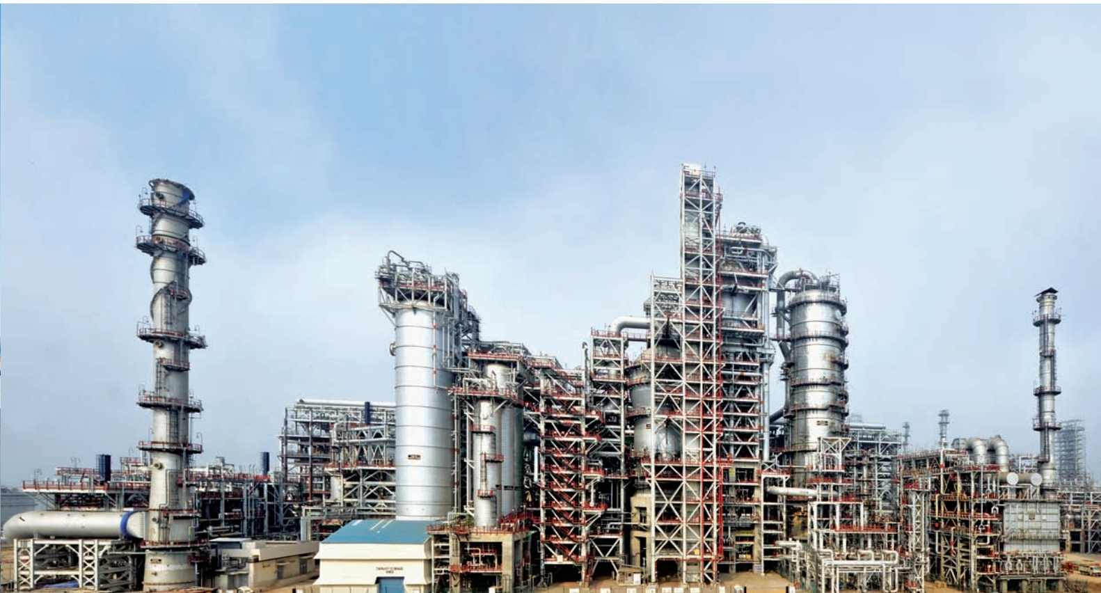
FCC Reactor Regenerator for Indian Oil Corporation Limited at Paradip Refinery, India
