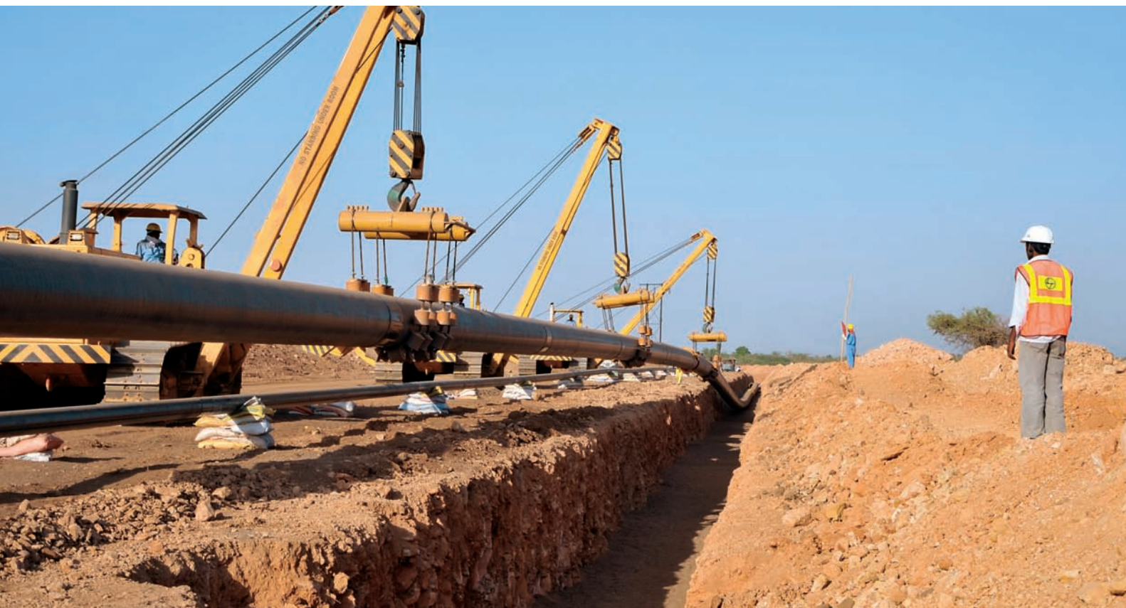
Laying of the world's longest heated and insulated crude oil pipeline in India from Barmer to Bhogat 24" x 619 km crude oil pipeline and 8" x 527 km natural gas pipeline
