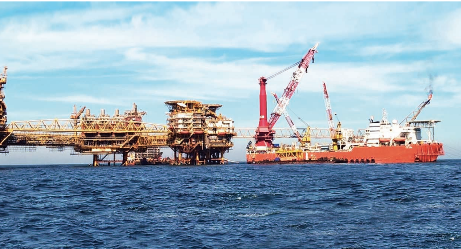
LTS 3000, a heavy lift-cum-pipelay vessel working for Vasai East Development Project of ONGC, India. The vessel gives an edge to the Company for installation of structures and pipelines for its offshore projects
