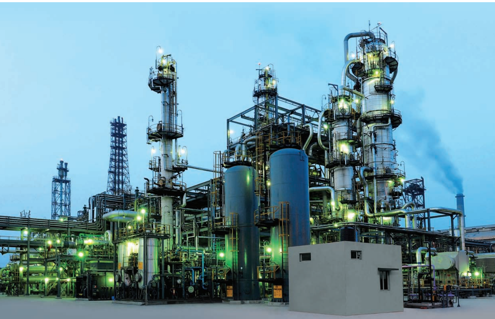
900 TPD Ammonia plant of National Fertilizers Limited, Panipat
