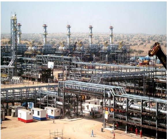
Mangala Process Terminal for Cairn India at Barmer in Rajasthan
