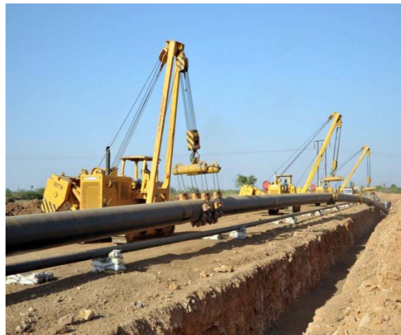
World's longest & PUF insulated waxy crude pipeline (24" dia. x 592 km) for Cairn India
